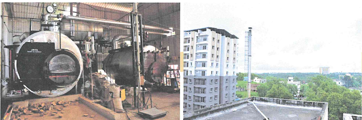
Fig 3. Boiler and Chimney
