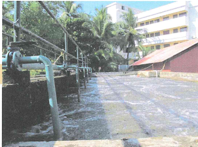
Fig 2. Sewage treatment plant
