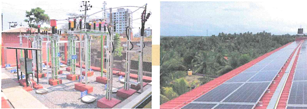
Fig 4. Power station and Solar panels
